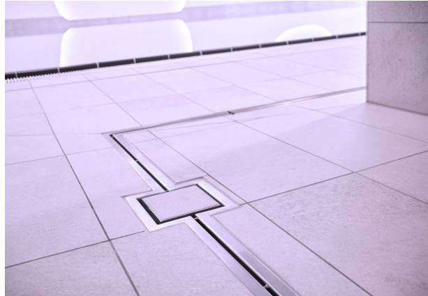
Around 180 metres of custom-made and extra-flat slotted channels from KESSEL in the pool surround. (Source: KESSEL)
